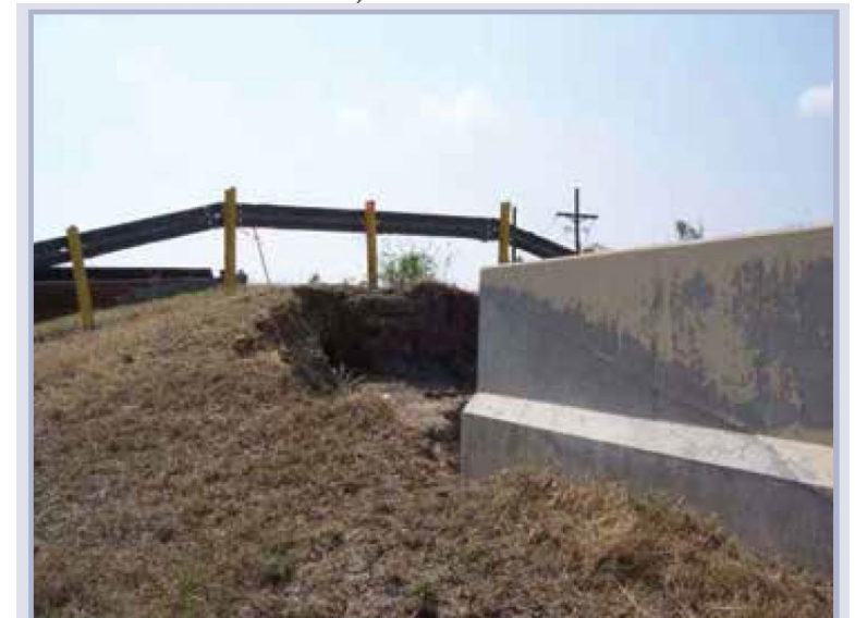
Figure 9.65 New Orleans levee scour at transition with a flood wall (courtesy USACE)
