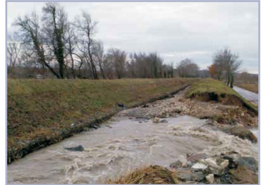
Figure 3.171 External erosion of the landward side (courtesy G Degoutte, Irstea)
