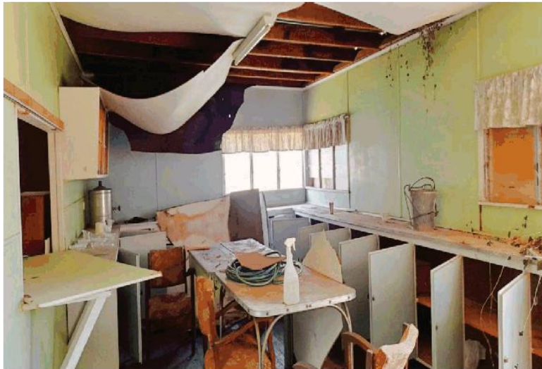
Hall Kitchenette showing roof lining collapse.
