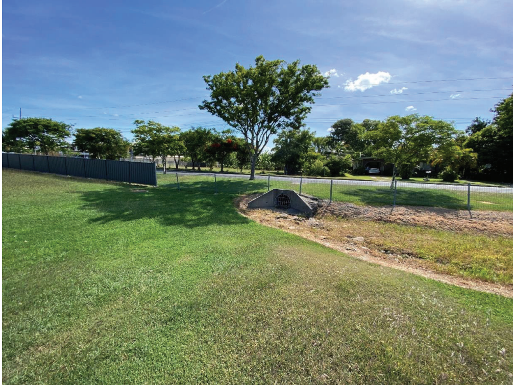
The stormwater headwall that captures stormwater discharge from the age care facilities underground stormwater drainage network
