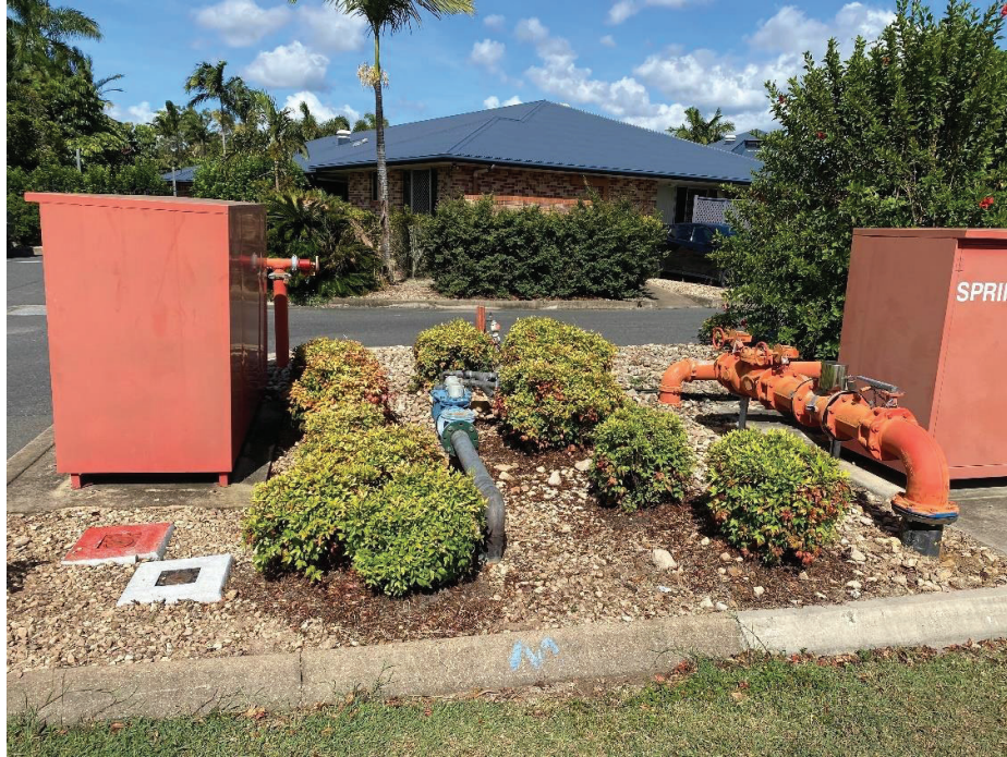
Age care facility water meter along Withers Street
