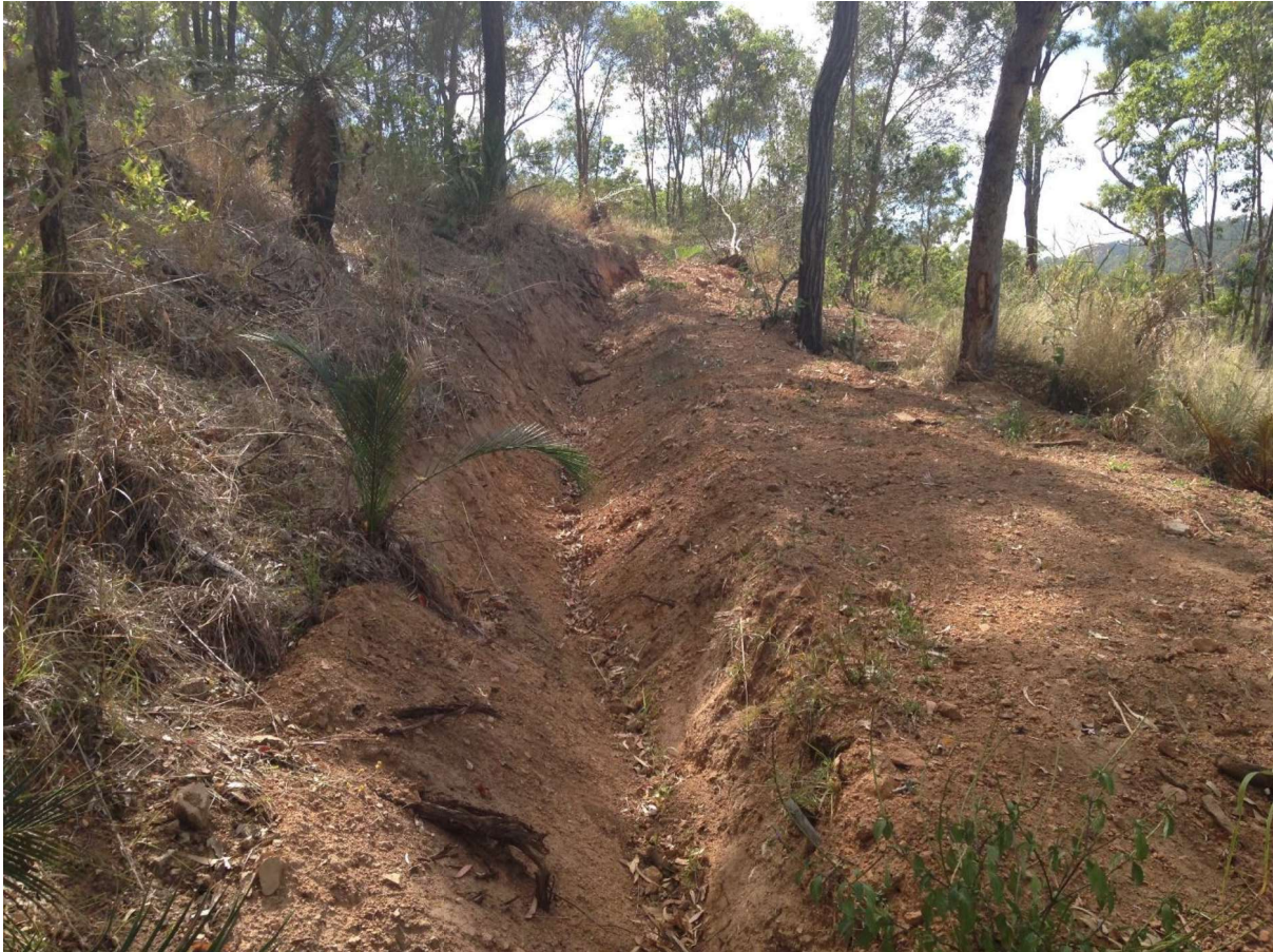
Figure 3. Unauthorised earthworks on Lot 1 RP4444. Open drain structure. Note Macrozamia miquelii left undamaged at left of drain, and Lantana camara at bottom right of image.
