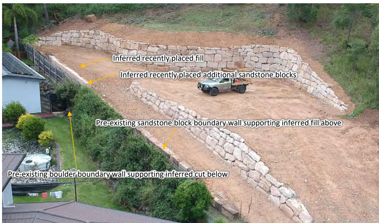
Figure 3: Image of site showing inferred recently placed sandstone blocks and fill in northwestern part
