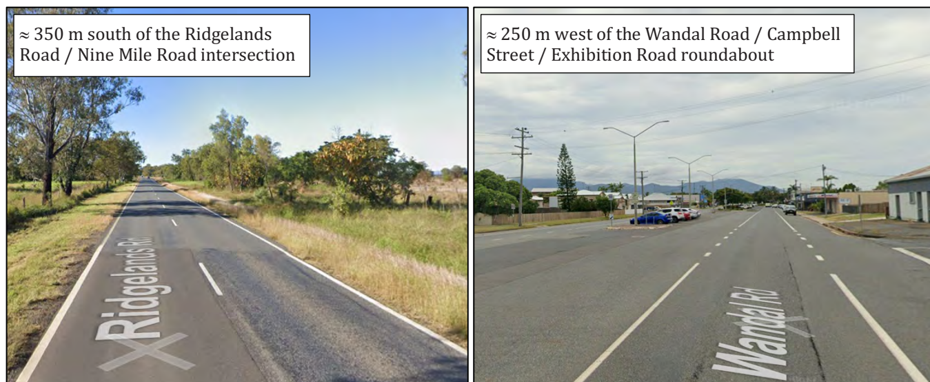
Figure 2.4: Ridgeland Road pavement conditions in year 2022 at various locations [Source: Google Street View]
