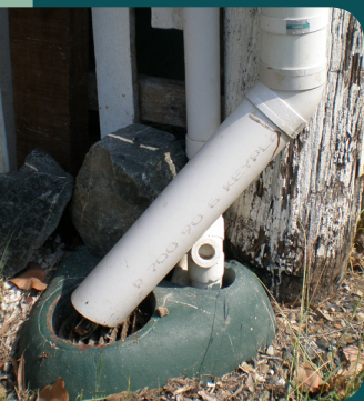
Illegal connection pictured - downpipe pointing to an overflow relief gully
