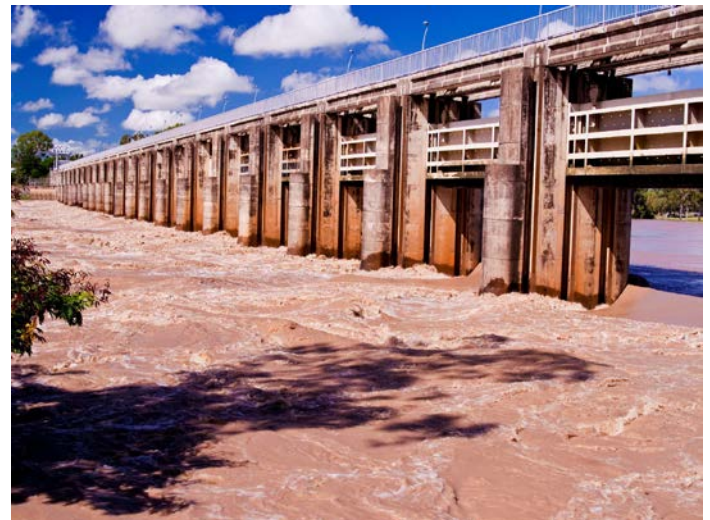
The Fitzroy Barrage is shown during a major flood event. The Barrage gates can be seen raised well above the passing flood water.
