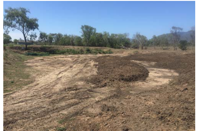
Fitzroy River Water's biosolids storage area at the South Rockhampton Sewage Treatment Plant
