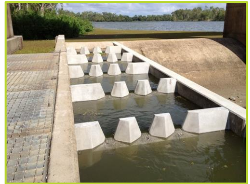
The new Fish Ladder at the Fitzroy River Barrage – a joint Fitzroy Basin Association and Fitzroy River Water project under the Federal Government's Reef Programme.
